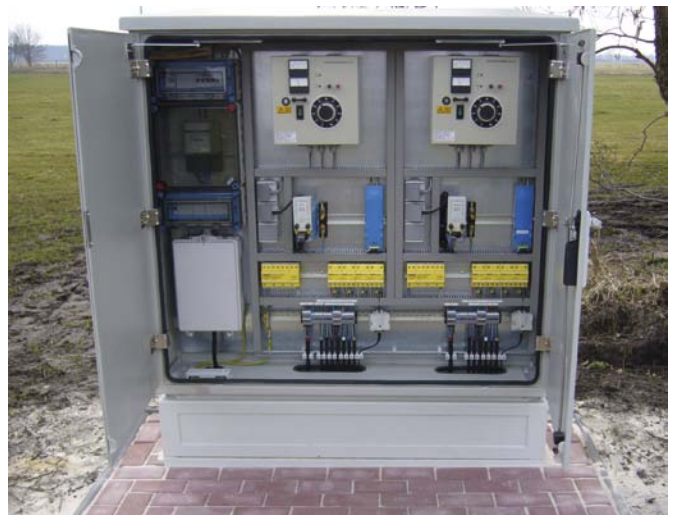
Protection of a rectifier substation (LAF Brachwitz)
